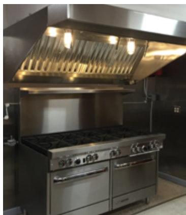
The new stove at the Dwelling Place!
